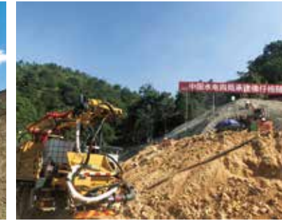
HPC30V混凝土喷浆车 福建泉州佛仔格隧道 HPC30V truck-mounted concrete spraying machine Fuozige tunnel in Quanzhou, Fujian
