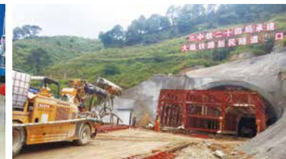
HPS30V混凝土喷射台车 云南大临铁路新民隧道 HPS30V concrete spraying trolley Xinmin tunnel along Dalin railway in Yunnan
