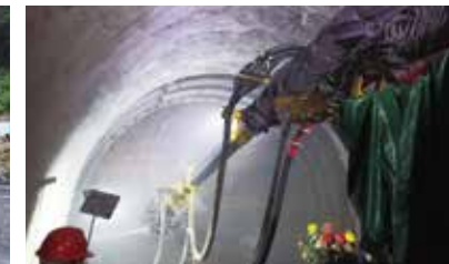
HPC30V混凝土喷浆车 济南绕城高速二环舜玉路地下隧道 HPC30V truck-mounted concrete spraying machine Shunyulu underground tunnel along Second Ring Road of Jinan Ring Expressway
